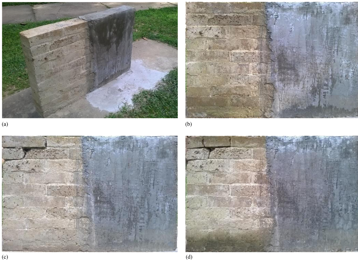
Fig. 8. Durability study of a CSEB masonry wall exposed to Baton Rouge weather: (a) wall after construction; (b) wall after 1 month of exposure; (c) wall after 3 months of exposure; and (d) wall after 6 months of exposure
